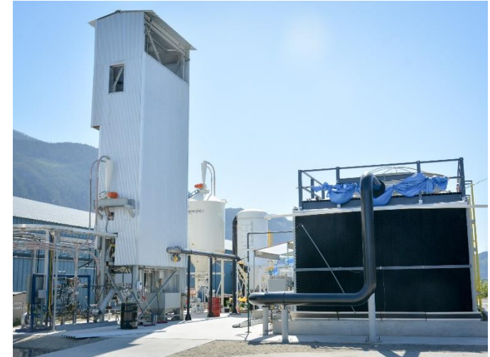
2015-2018: End-to-End Pilot Plant
