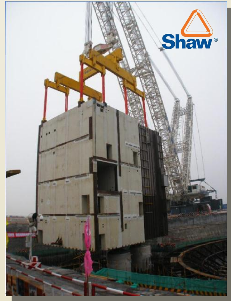
AP1000 reactor auxiliary building (China installation) same size as entire EM 2 module pair
